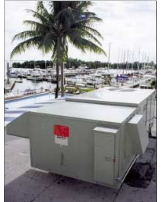
Figure 2. The SEMCO FV-2000 fresh-air ventilation module is bolted to the 7.5-ton Trane Voyager rooftop system.
