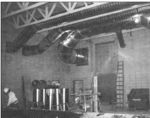
Round ductwork provided substantial noise reduction and first-cost savings compared to rectangular duct.
