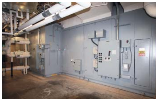
Four custom-built energy-recovery ventilating units enabled Navy Federal Credit Union to earn LEED points.
