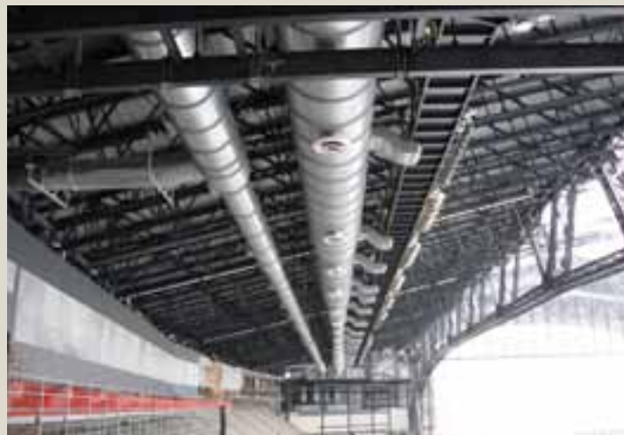
This spiral ductwork was installed at the Lucas Oil Stadium, the home field for the Indianapolis Colts. Some of the ductwork was as large as 118 inches in diameter.
